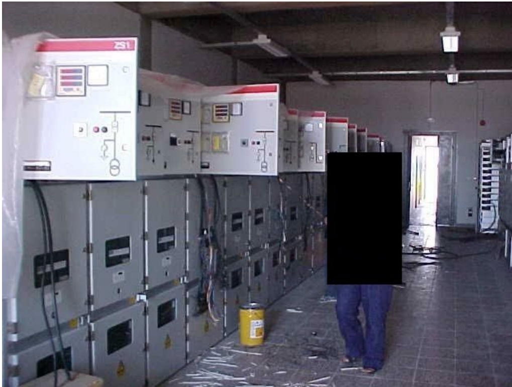
Pictorial representation of HT Panels with control door open and Engineer without helmet
